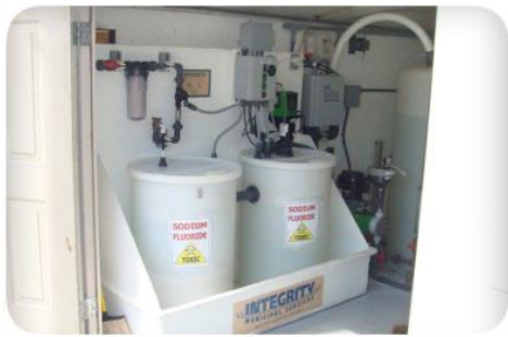
Park Water Company, CA
