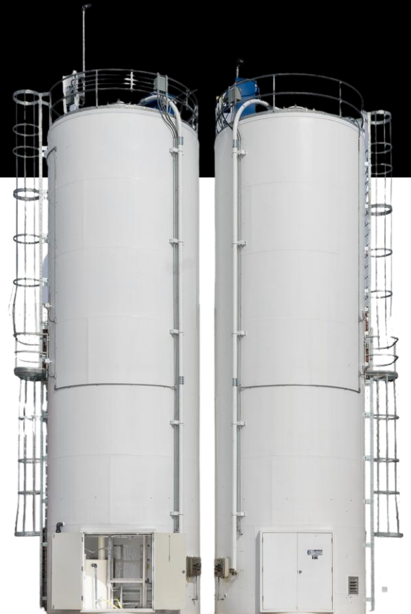
Bulk Chemical Storage and Feed System
