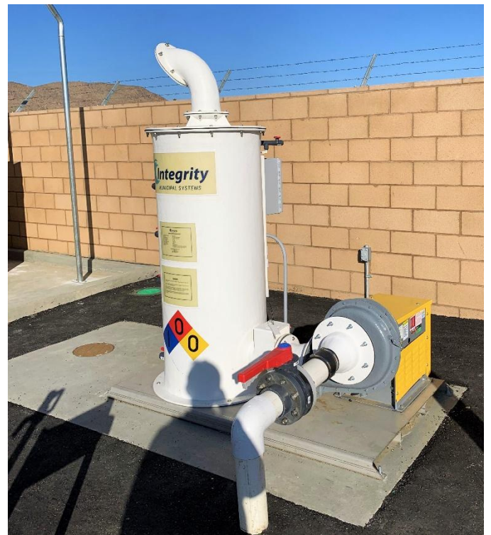
IMS Modular Carbon Odor Control System (MCS-0200) installed at the Barron Pump Station at the Intersection of Barron Ave & Yucca Mesa Rd
